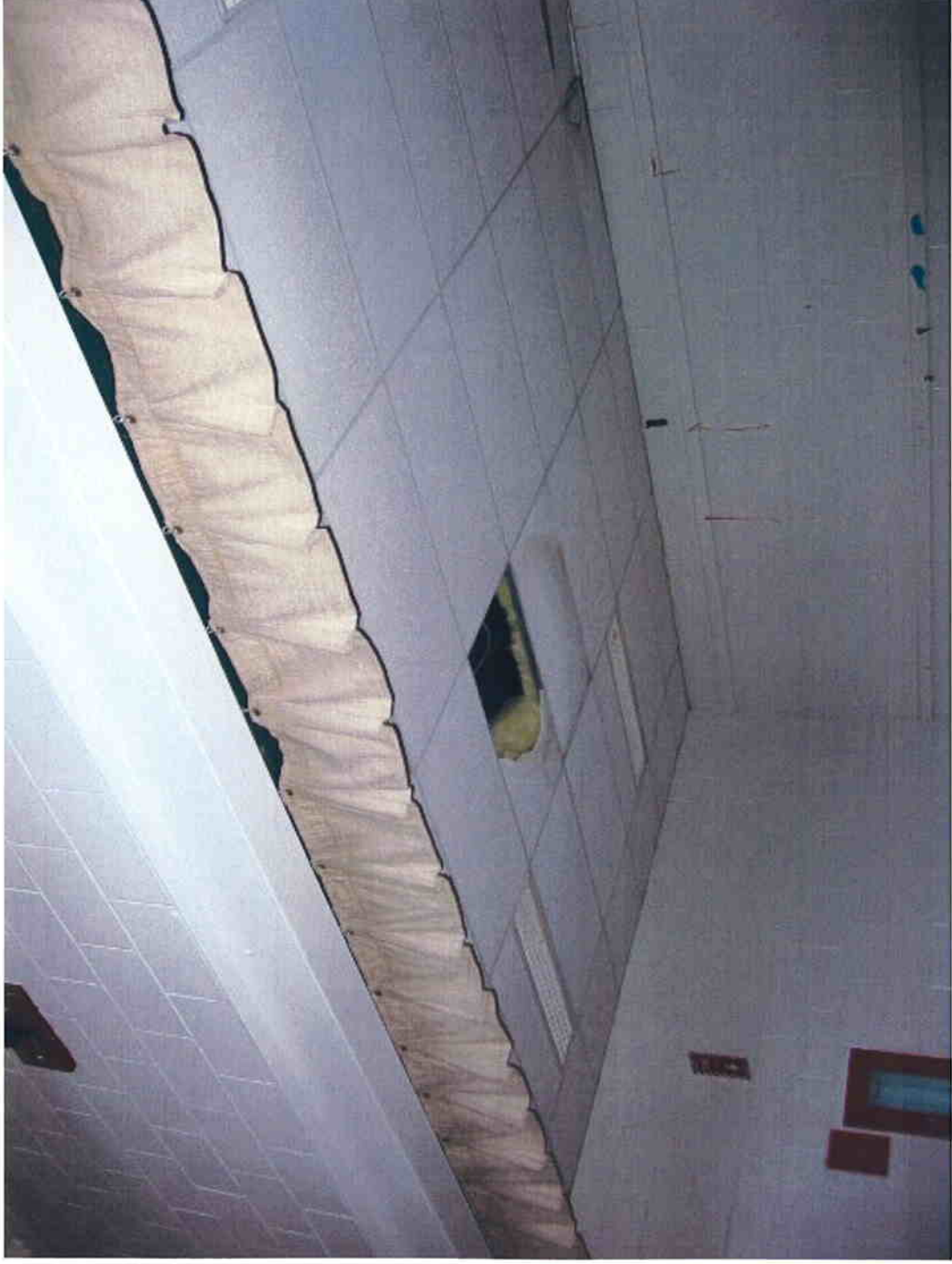
Leaky Roof Water Damage Over Stage - Groton Heights Elementary School
