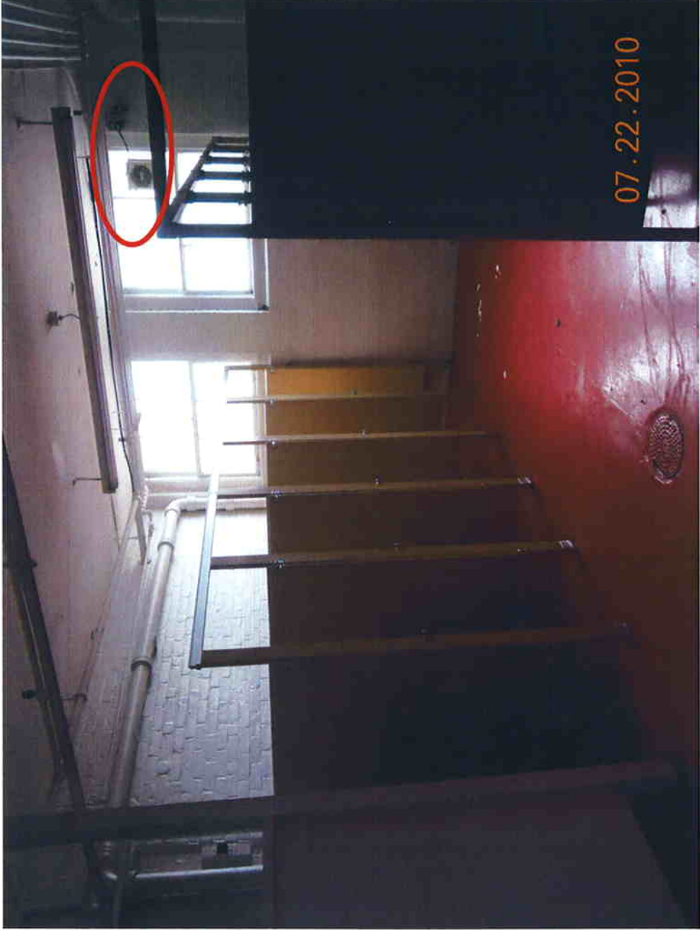
Bathroom with Ventilation (in red oval) - Groton Heights Elementary School
