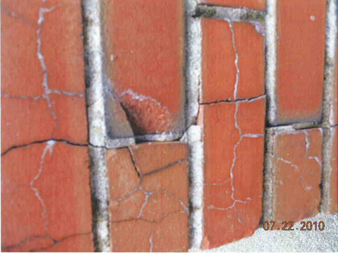
Structural Cracks in Exterior - Groton Heights Elementary School
