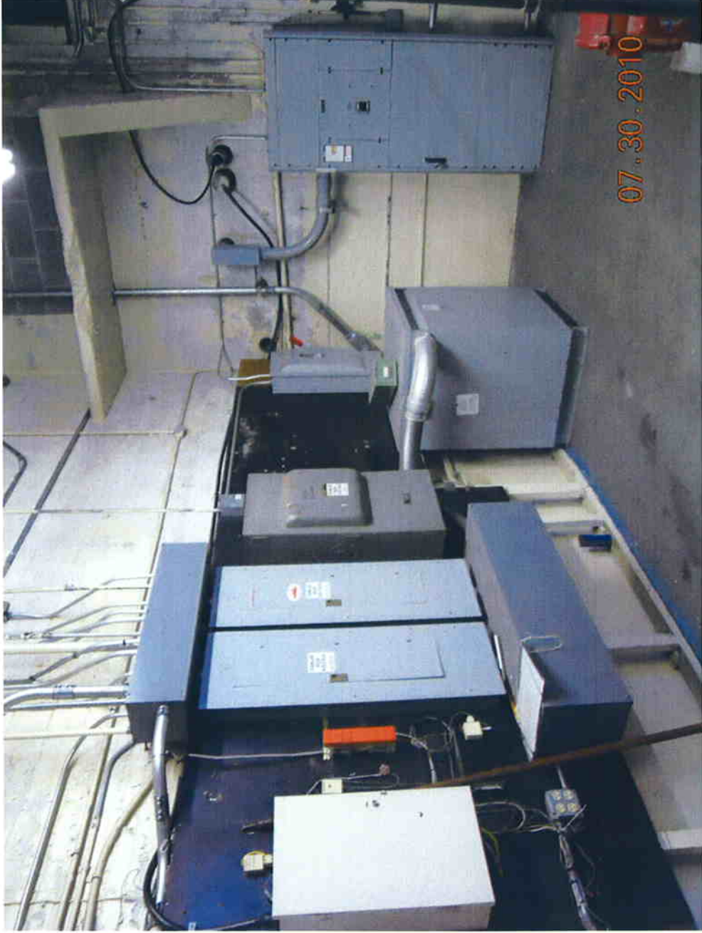
Electrical System - Groton Heights Elementary School
