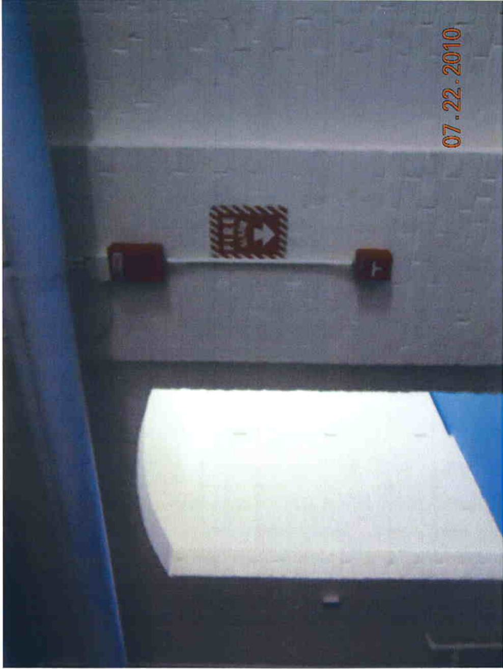
Fire Alarm System - Groton Heights Elementary School
