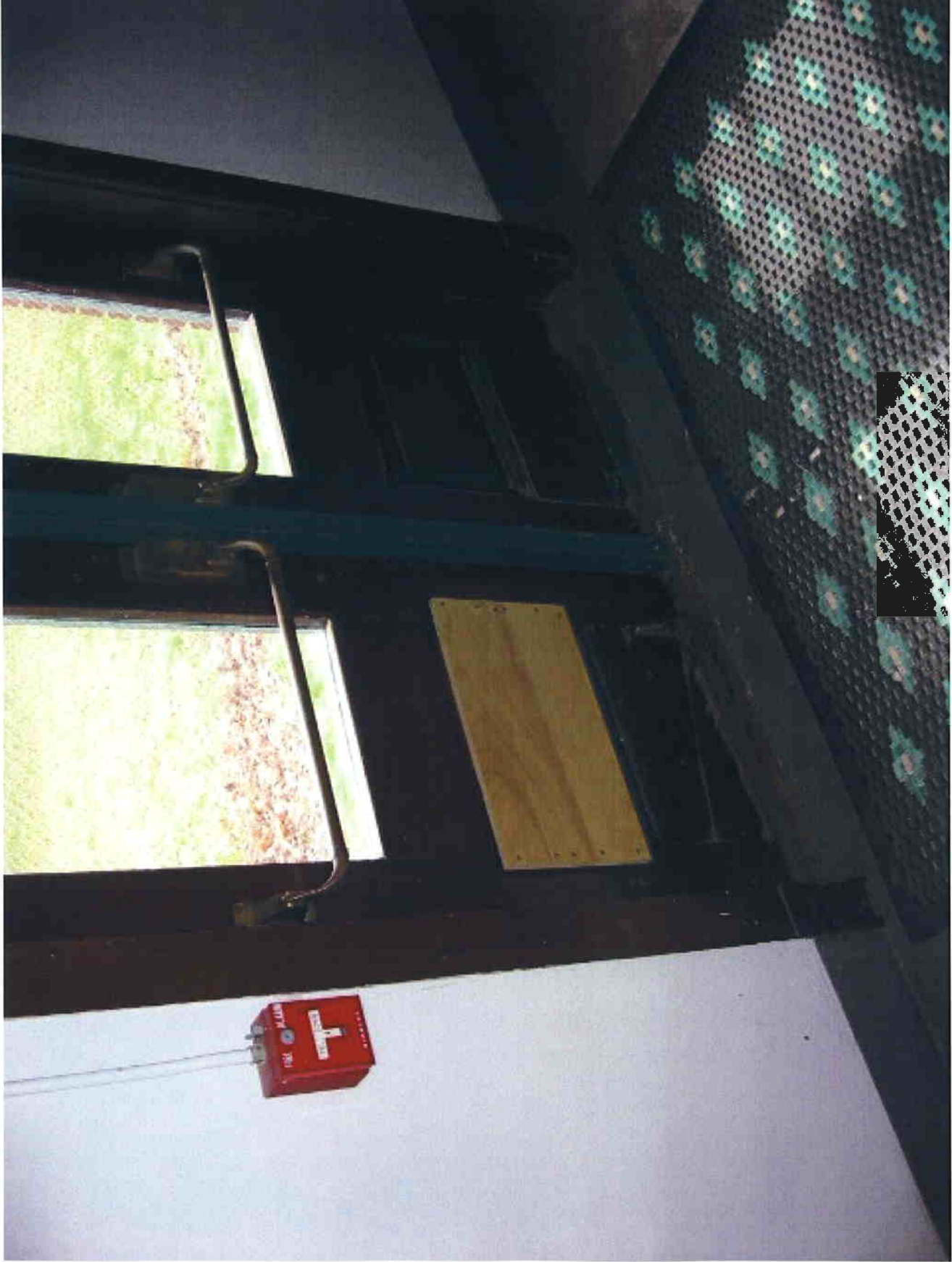
Side Entrance Doors with Vandalism – Groton Heights Elementary School
