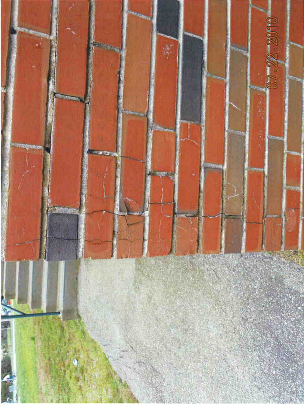
Structural Cracks in Exterior - Groton Heights Elementary School
