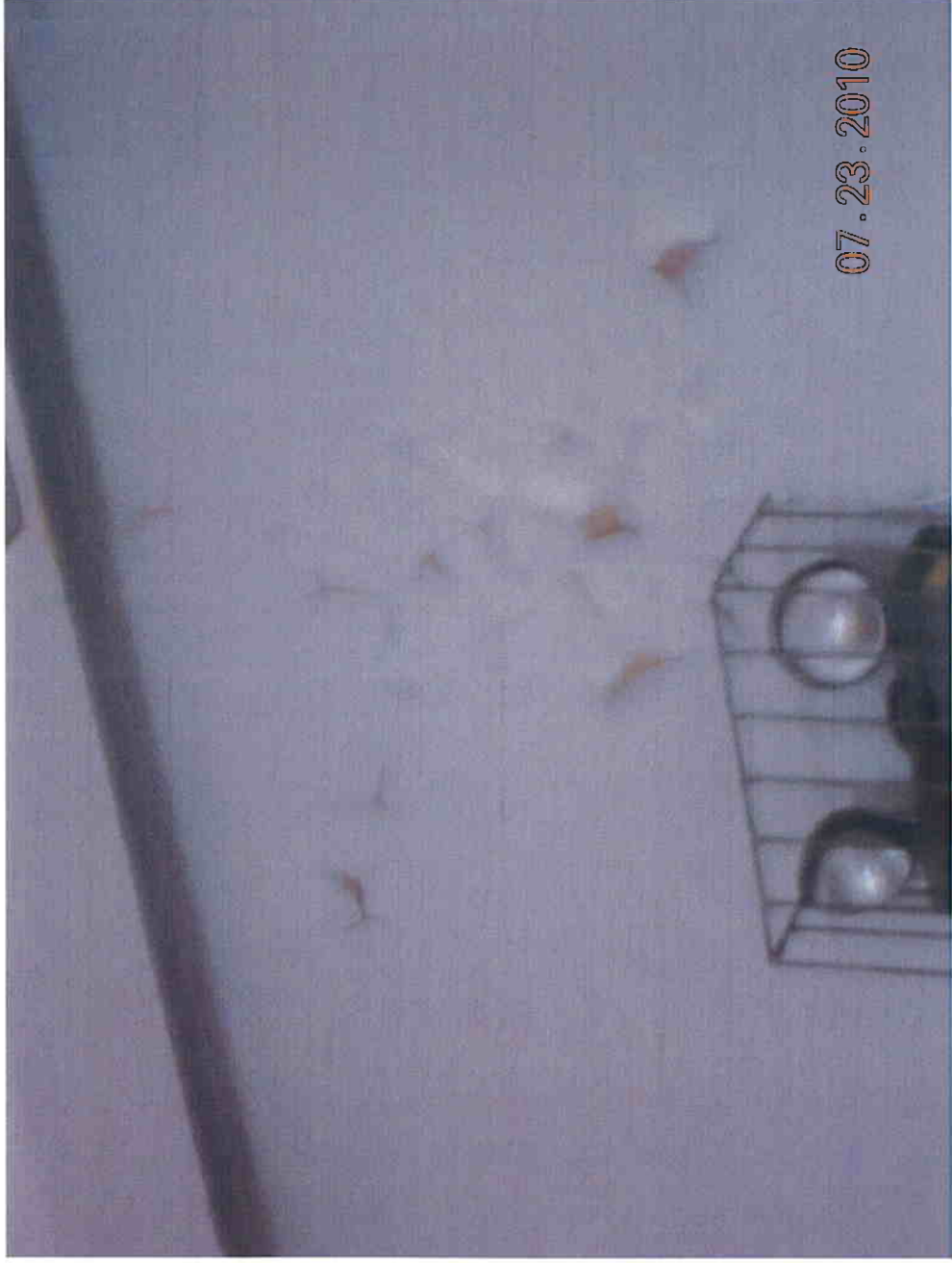
Emergency Lighting - Groton Heights Elementary School
