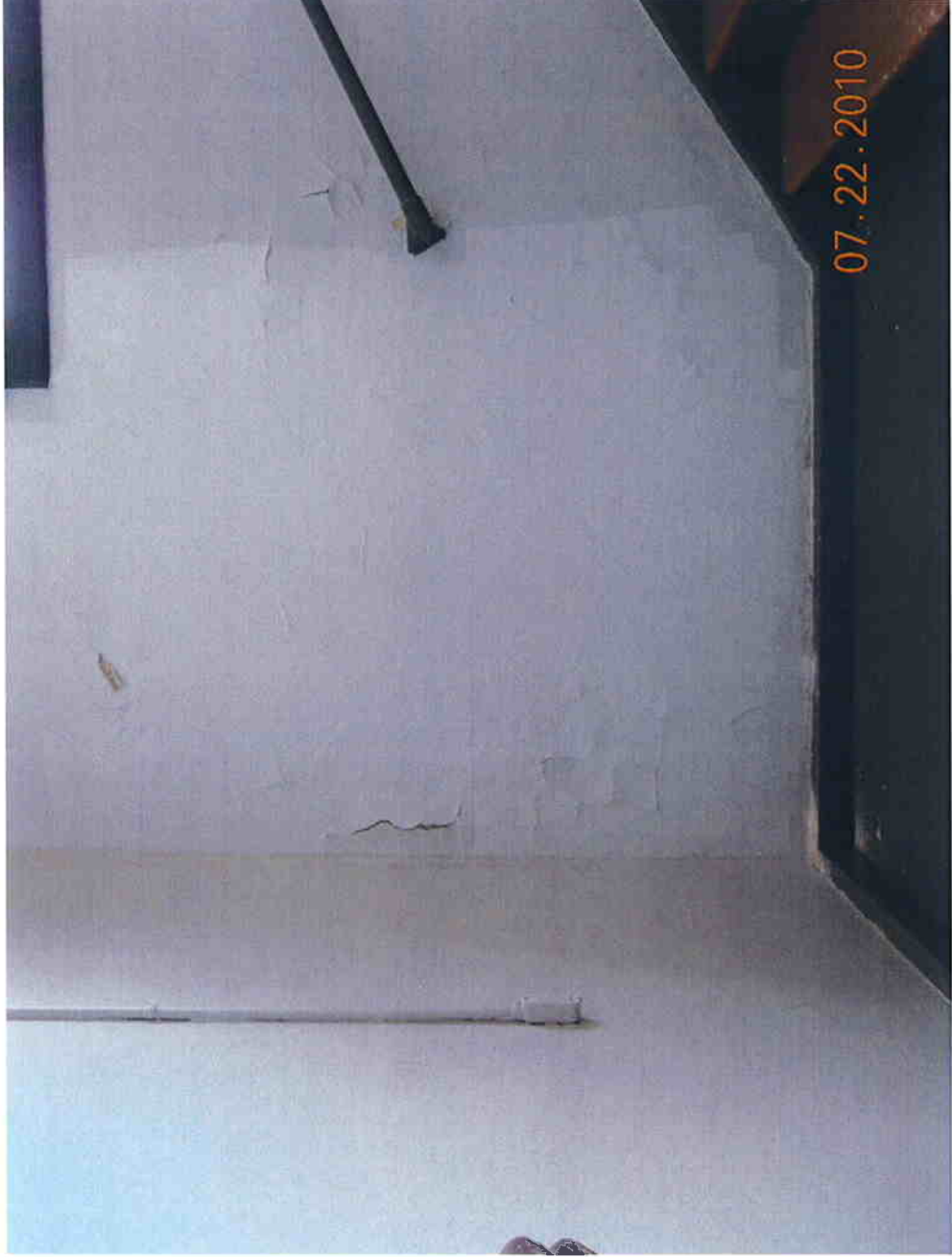
Failing Paint - Groton Heights Elementary School
