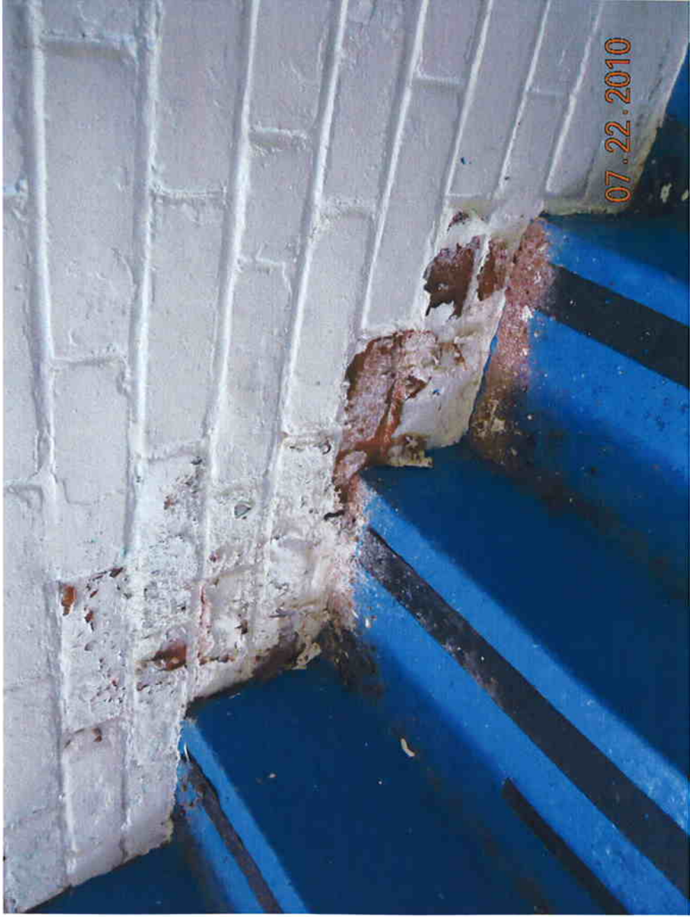
Failing Paint - Groton Heights Elementary School
