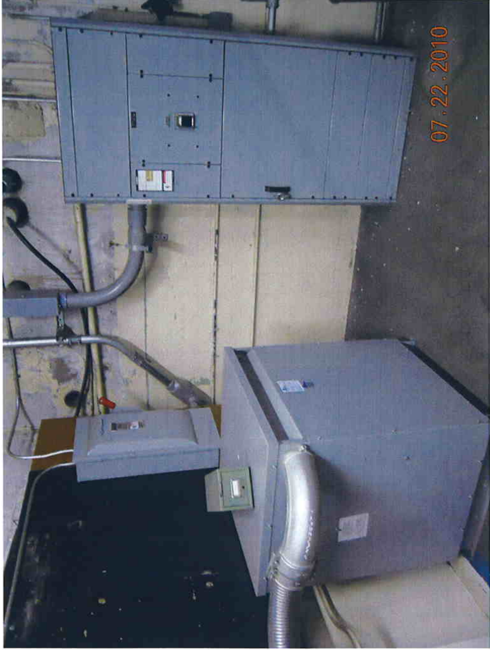
Power Conditioning System - Groton Heights Elementary School
