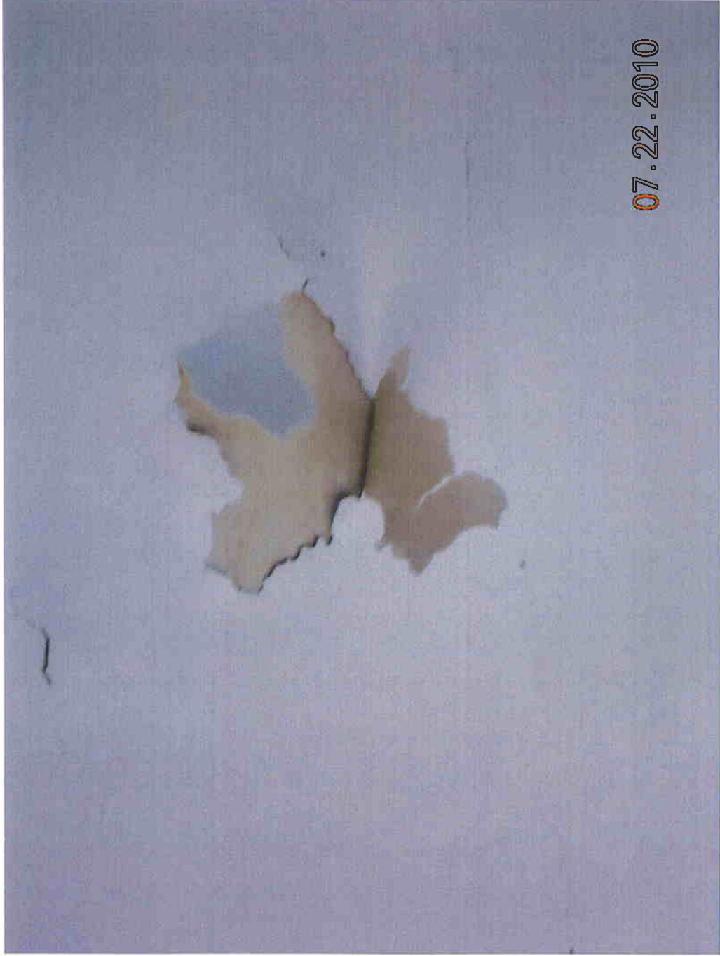
Failing Paint - Groton Heights Elementary School
