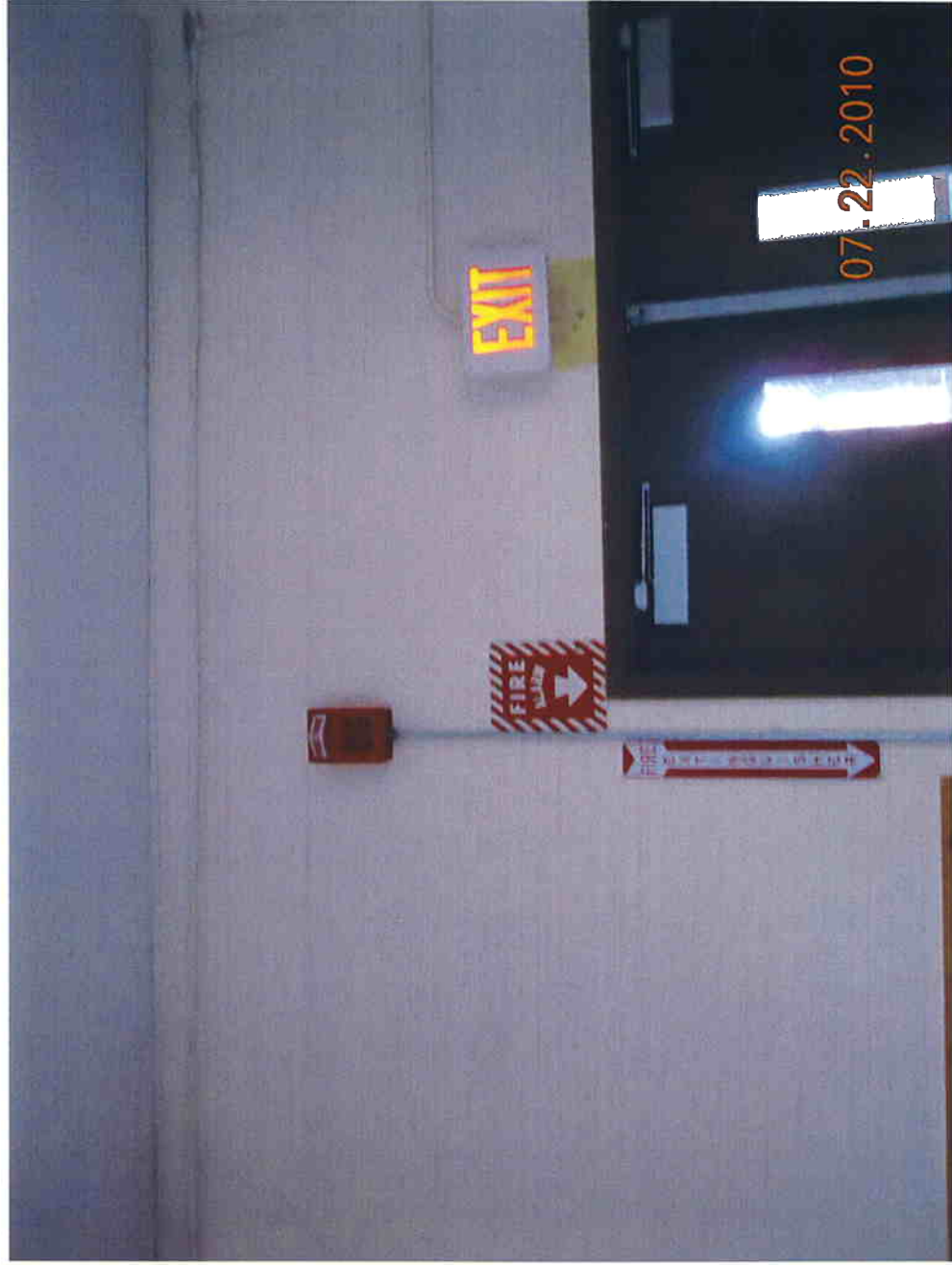
Fire Alarm System - Groton Heights Elementary School
