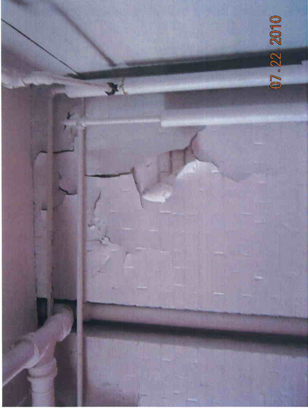
Failing Paint - Groton Heights Elementary School
