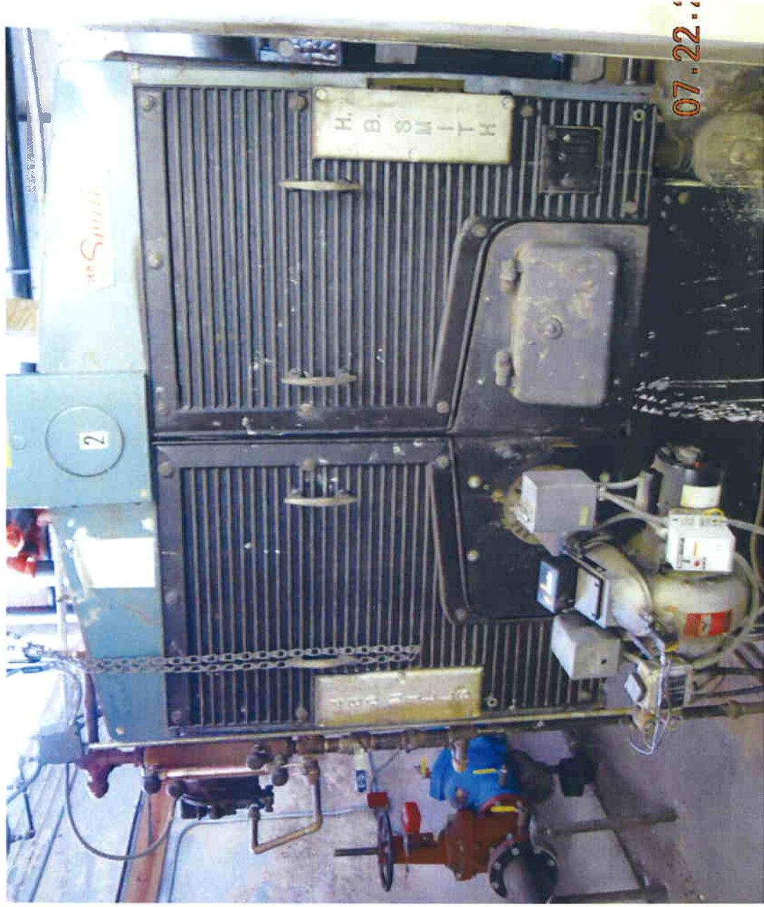
HB Smith Boiler #2 - Groton Heights Elementary School
